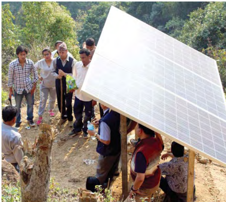
Monitoring visit by WASH team of Caritas Nepal. Solar panels seen on top
